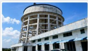
Water Treatment Plant Project Site
